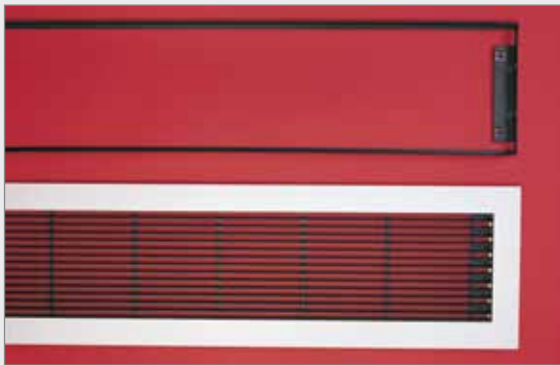
Loose grille & frame
