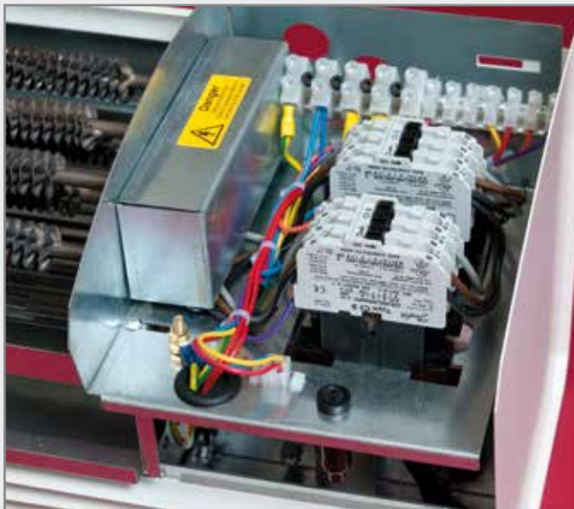
Electrical connections box
